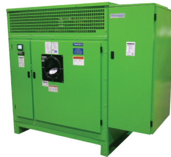
Above: Energy Station TX™, 1000 kVA, with output breakers (right side), integrated Cyberhawk™ monitoring, rotatable IR Port and hinged door options
